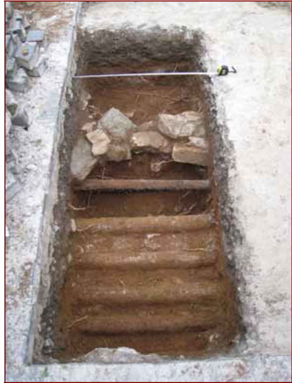
Figure 3: A view to the north of trench E showing the gas pipes (007) in the foreground and the power cable and its rock backfill (004) beyond them. 1m scale
