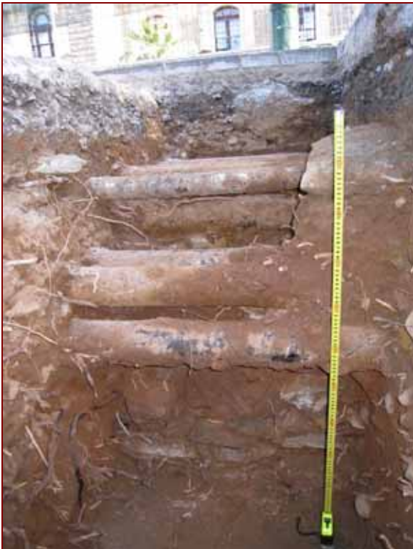
Figure 5: A view facing south of the wall in Trench E. Note the proximity of the service pipes to the wall. 1m scale
